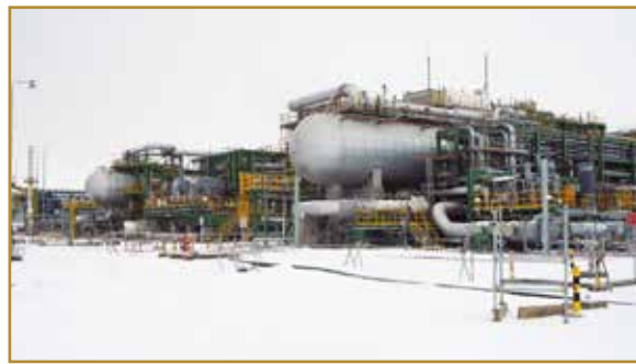
Future Growth Project-3GP ME&I - Power Generation, Reception Area & Pressure Boost Facility, Kazakhstan
